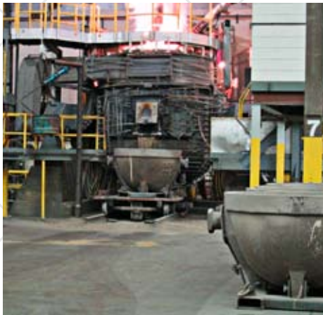
Electric arc furnace technology helps to maximize recovery of precious metals in spent catalysts.
