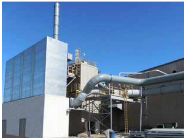
Figure 5. Minimizing harmful atmospheric emissions is both mandatory and critical. Baghouses such as this prevent discharge of noxious, toxic, or annoying fumes or odors, while capturing remaining precious metal particulates prior to atmospheric discharge.
