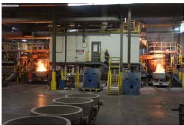
Figure 4. Slag from the dual electric arc furnaces—containing trace amounts of precious metals—is poured into slag pots which are set aside for cooling. The slag is shipped to SMC (Canada) Ltd. for subsequent refining. Dual electric arc furnaces double pyrometallurgical processing throughput to help assure maximum recovery of remaining PGMs in spent catalysts—including rhenium.
