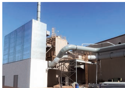
FIG. 3. The baghouse eliminates air pollution and captures precious metal particulates before discharge to atmosphere to ensure environmental law compliance.
